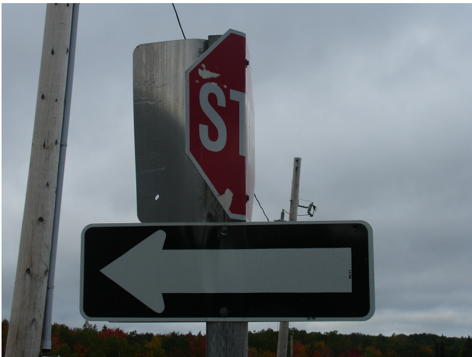
Figure 2: Damage to a Stop sign and No Entry sign (the back of which is visible) was probably caused by a snow plough. It has rendered the No Entry sign virtually impossible to read and has reduced the legibility of the Stop sign. Damage like this should be repaired immediately on discovery.
