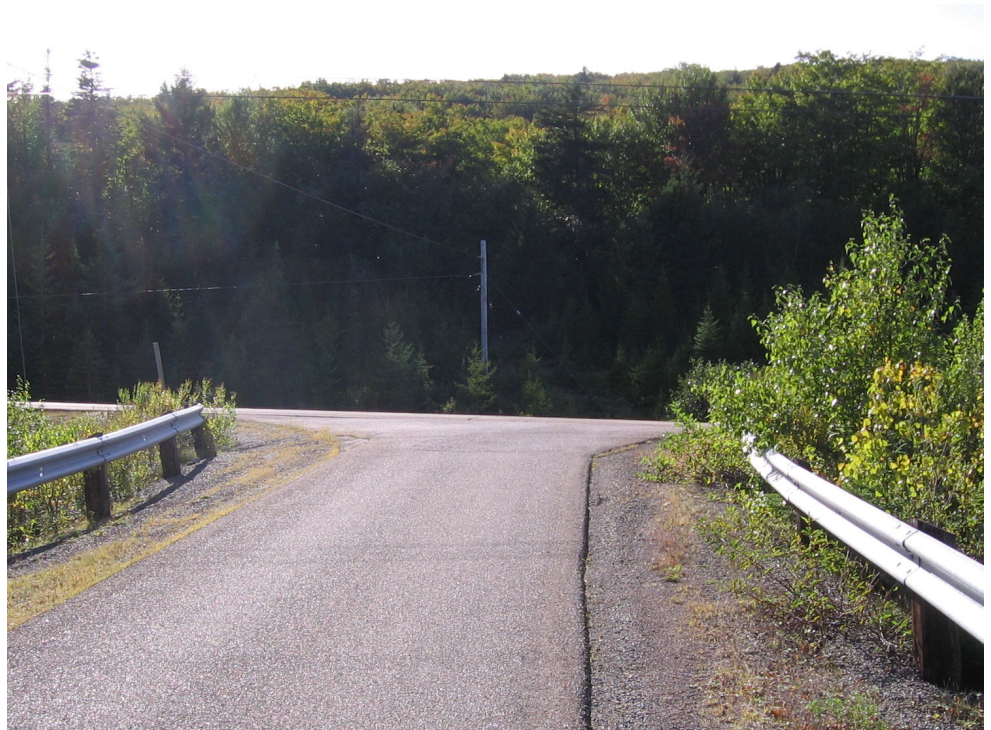
Figure 1: Example of inadequate signage. The intersection lacks stop controls either because the sign is missing or because it is obscured by overgrown vegetation. Some jurisdictions, including Saskatchewan, will permit this application on low-volume rural intersections.
